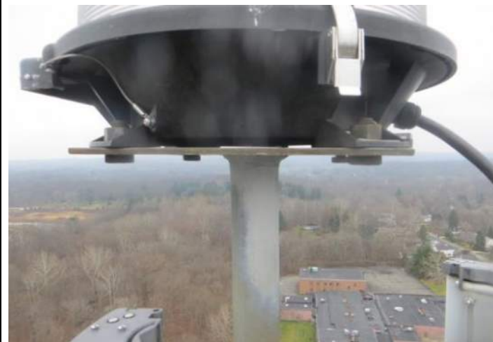
Full Side Ant. #4 Showing Downtilt Brackets(Level & Perpendicular)
