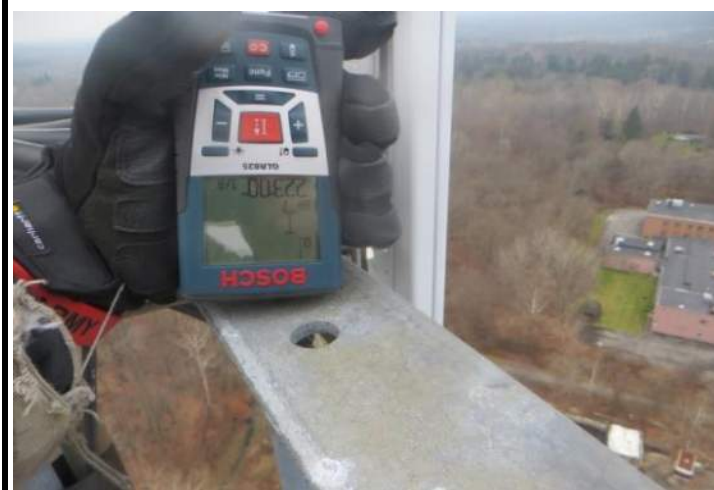
Centerline of Antenna #1 with Laser Tape
