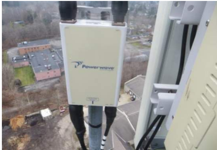
Back Side of Full TMA(s) (Level & Perpendicular)
