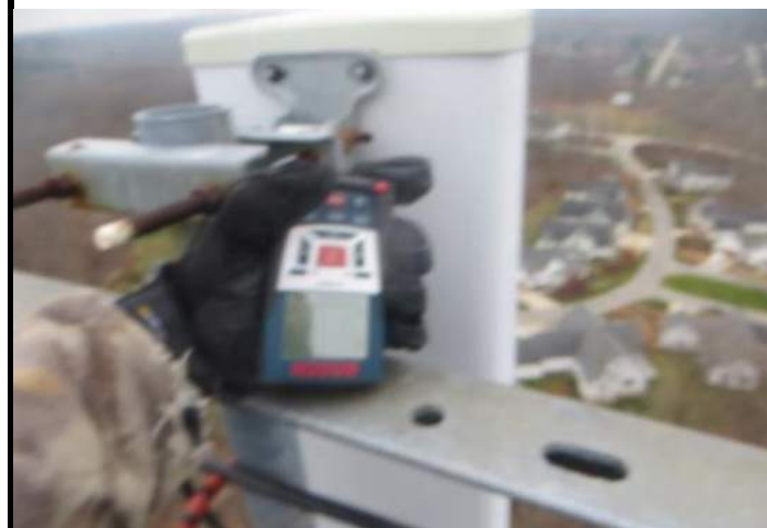
Centerline of Antenna #2 with Laser Tape
