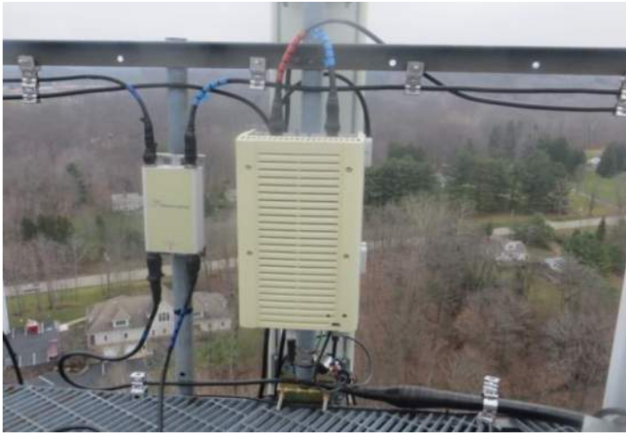
Back Side of Full RRH #1 (Level & Perpendicular)
