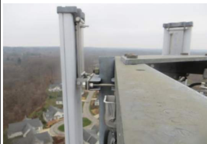
Full Side Ant. #1 Showing Downtilt Brackets(Level & Perpendicular)
