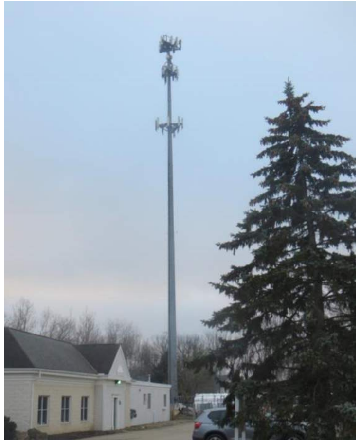
Full View Tower
