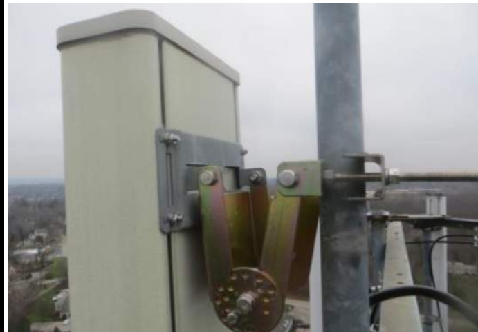
Full Side Ant. #3 Showing Downtilt Brackets(Level & Perpendicular)
