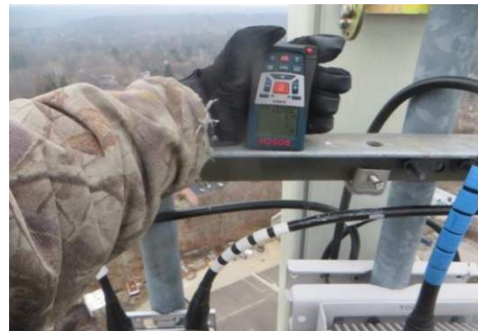
Centerline of Antenna #3 with Laser Tape
