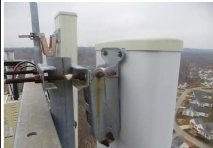
Full Side Ant. #2 Showing Downtilt Brackets(Level & Perpendicular)
