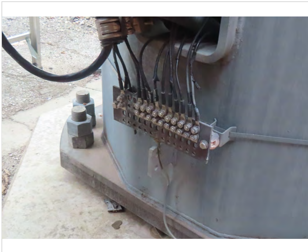
Photo 4: Lower Tower Ground Bar
