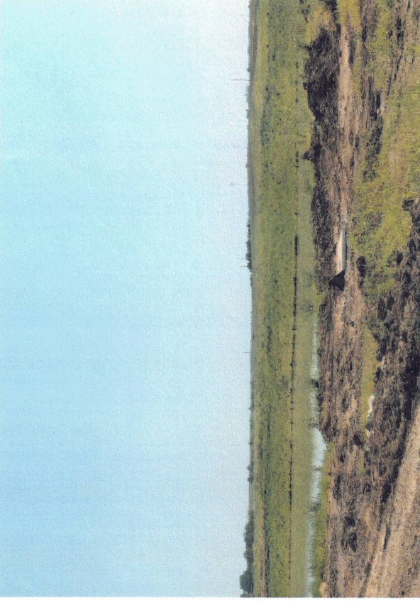
Photo 2 – Zone 1 – Inlet into Lake needs filter fabric repaired.
