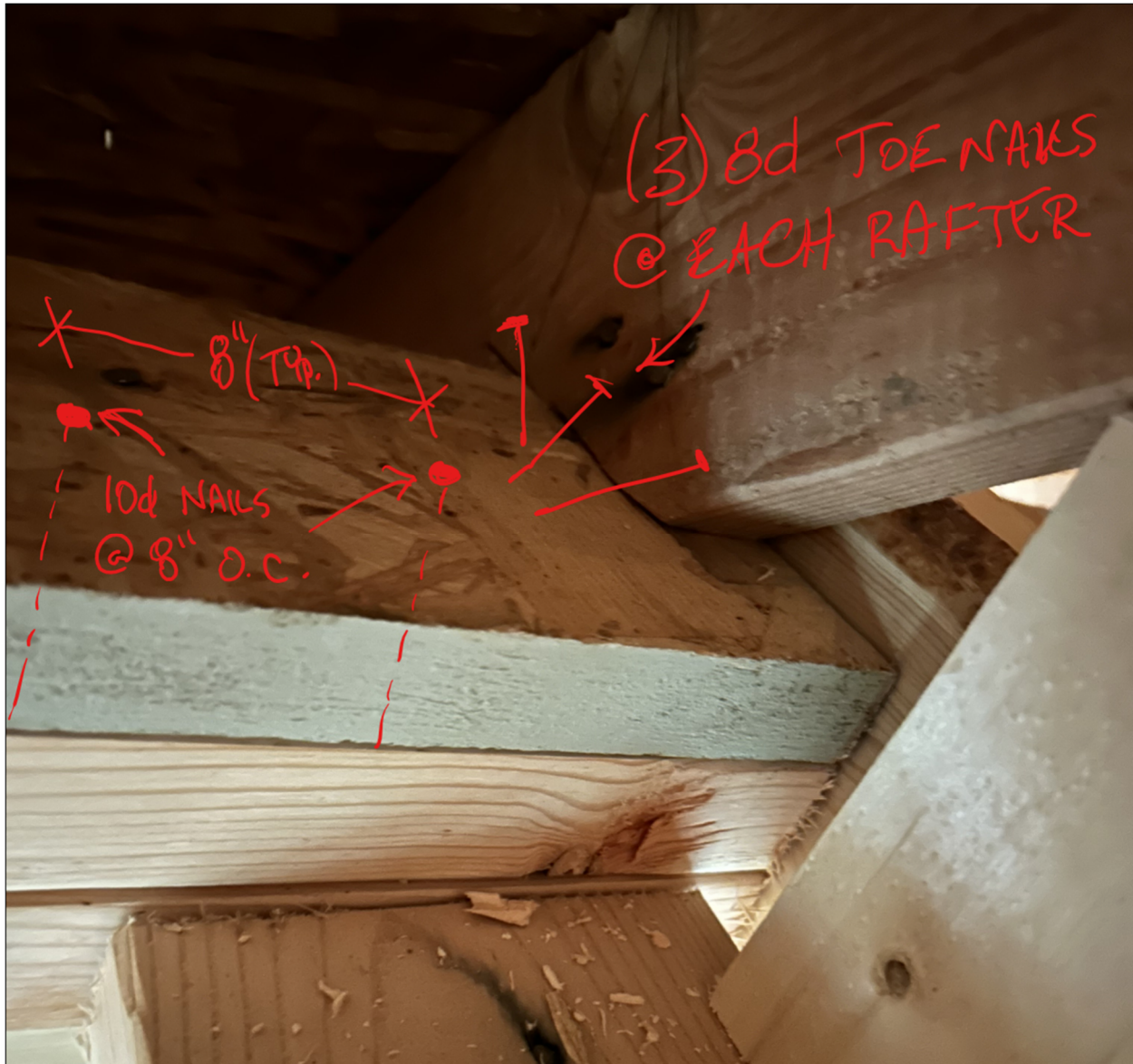
Photo #2 – fastening of rafters to vertical 2x4's and vertical 2x4's to ceiling joists
