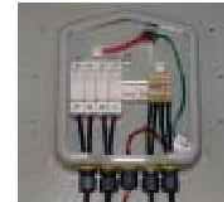
Model SD 0786-41, wired with Din Rail mounted fuse holders, terminal blocks and bus bars.
