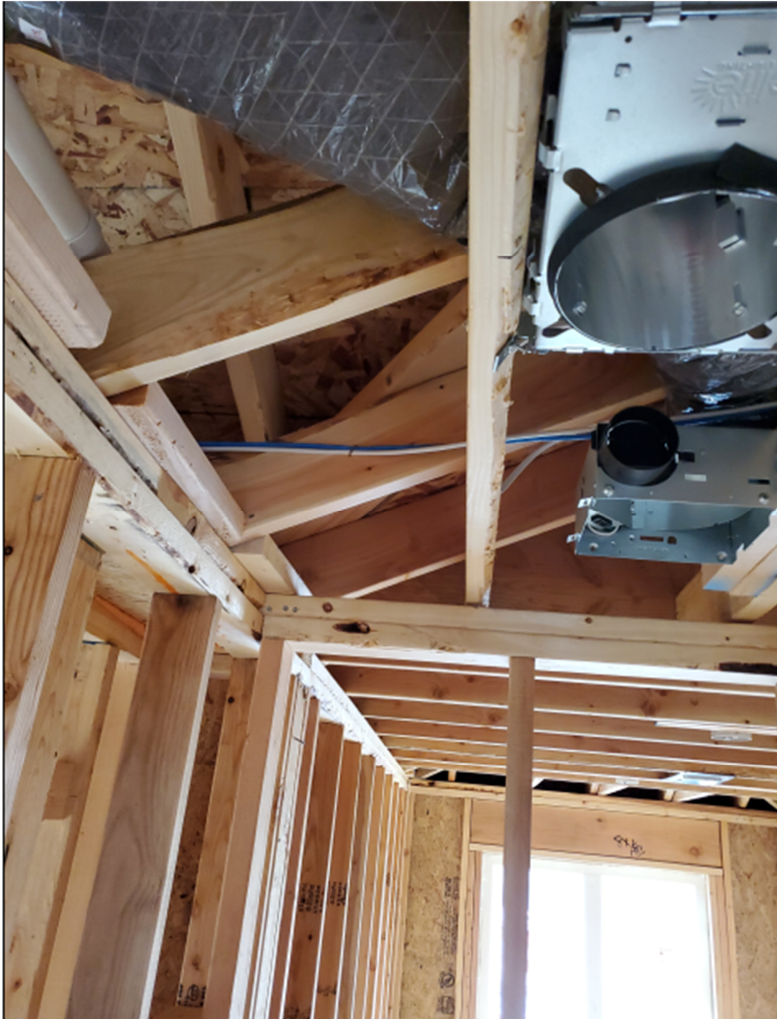
2034 Hook Farms Drive – rafters bearing on wall not shown as load-bearing on plans
