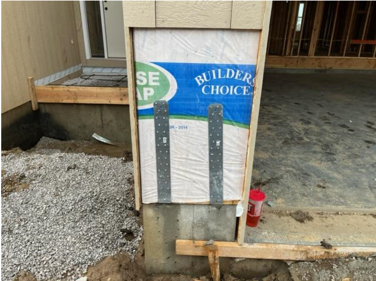
2614 SW Farmfield Road - Garage Portal Frame – Installed as PFH (with hold-down straps)
