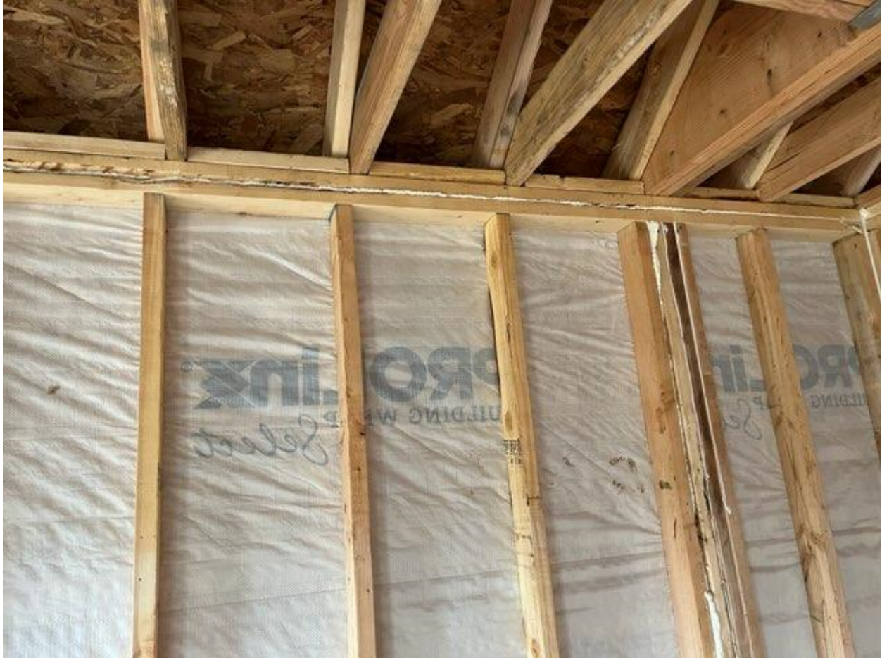
2614 SW Farmfield Road - Rafters Bearing on flat 2x blocks.
