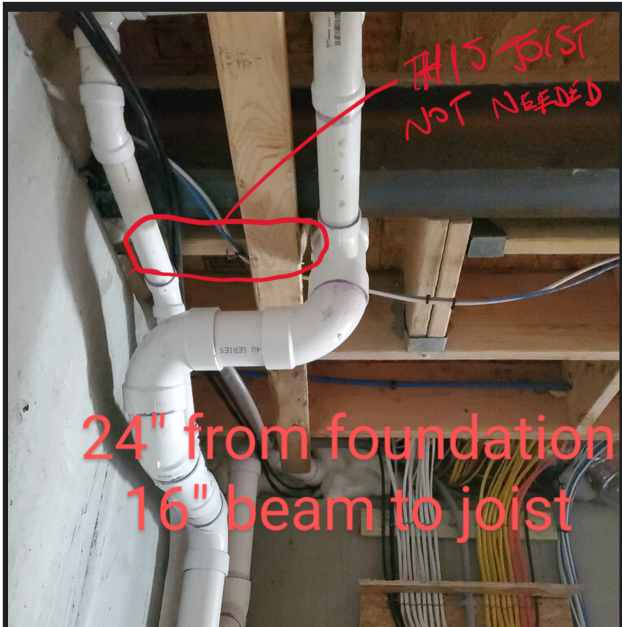
Picture of joist area in question
