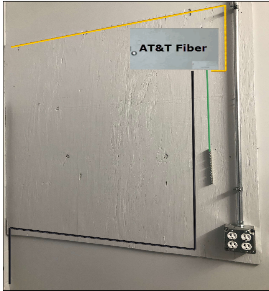
NORTH WALL TELCO ROOM
