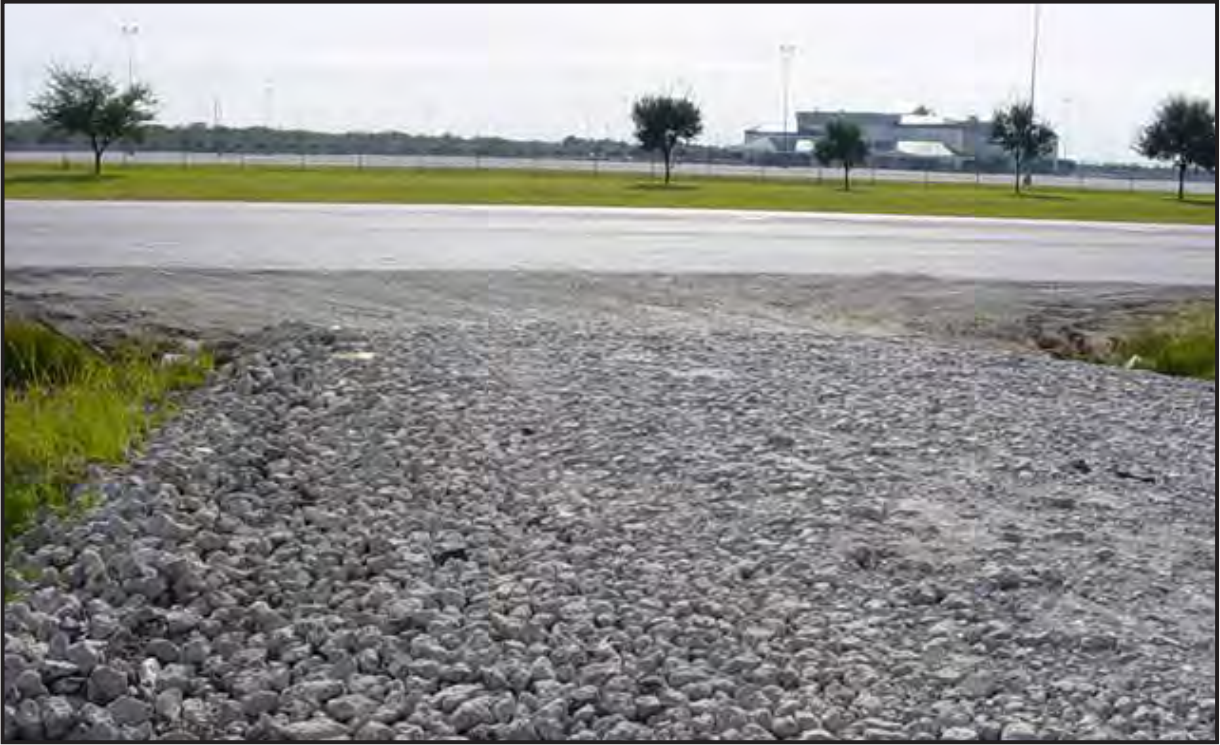
Figure 6.1 A temporary rock construction exit can reduce sediment and resulting safety hazards on public streets. This pad needs maintenance due to sediment filling the void spaces between the rocks making the rock exit pad ineffective. Source: ABC's of BMP's, LLC
