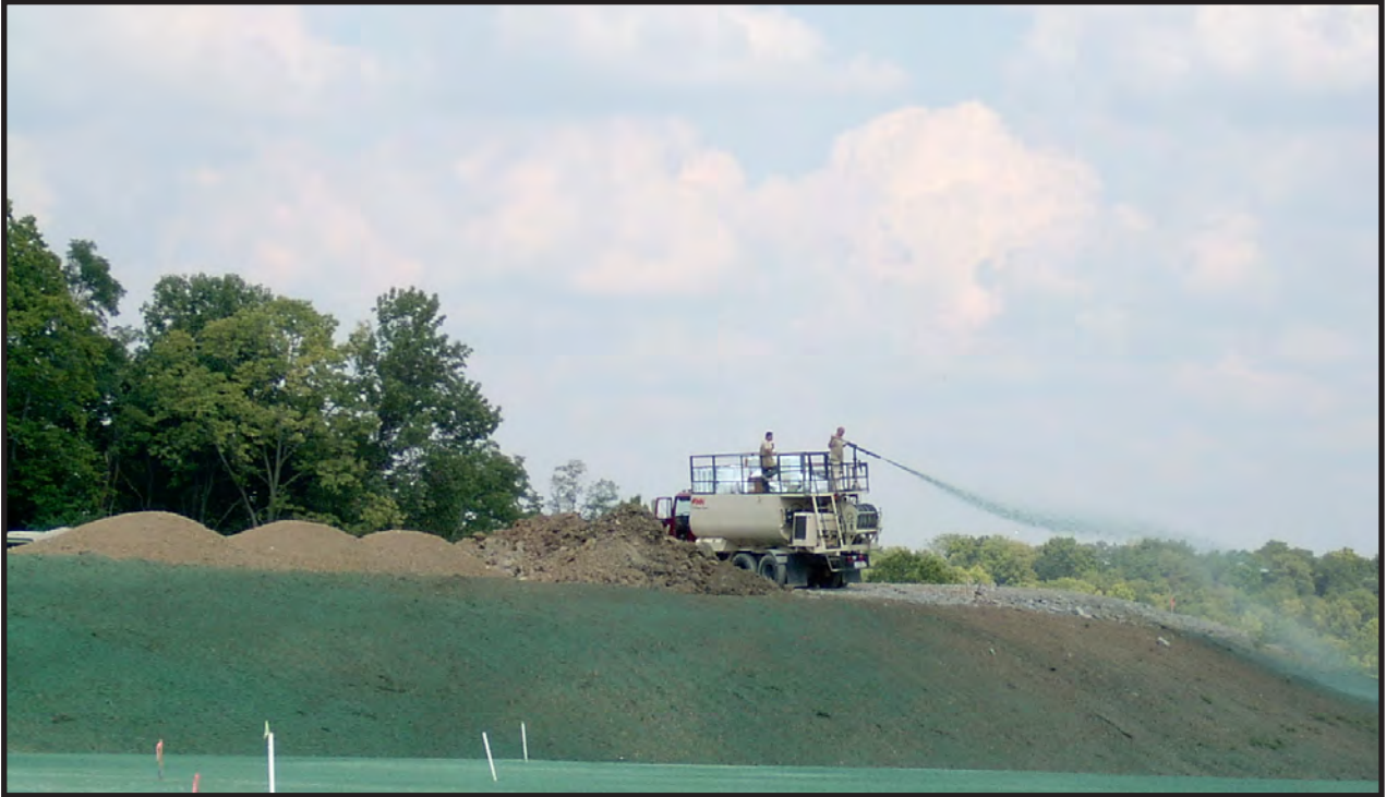
Figure 6.26: Hydroseeding over matt armoring on a steep slope to promote vegetation growth and prevent erosion. Source: Florida Erosion and Sediment Control Designer and Reviewer Manual , June 2007
