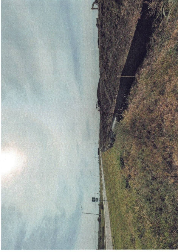
Photo 2 – Zone 1/Alora – Silt fence repairs needed, grading activities ongoing.
