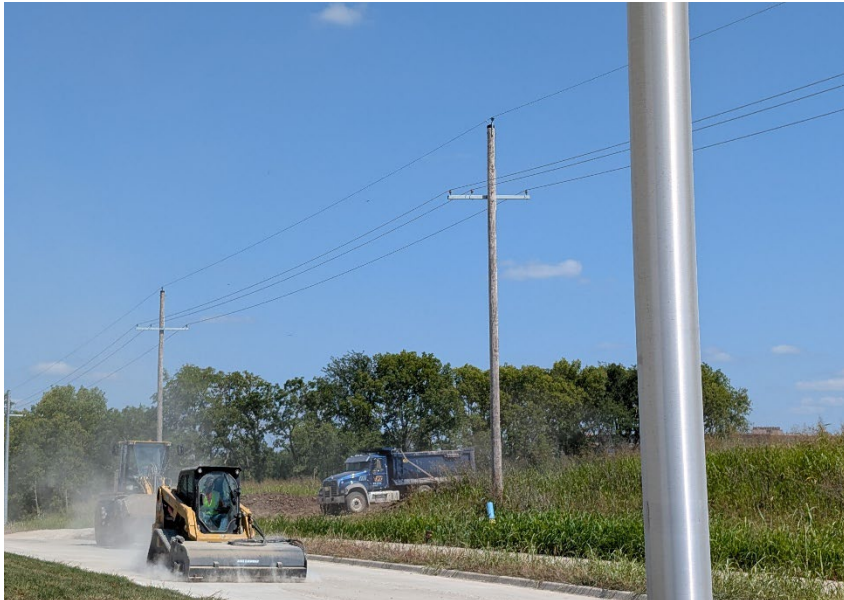
Photo 1 – Zone 1 & 3 – Recommend additional water trucks for dust.
